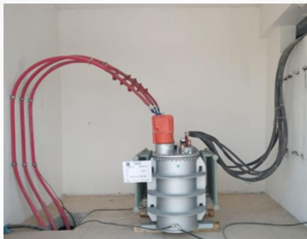
Figure 1: 50kVA, R410A gas insulated transformer in service.
