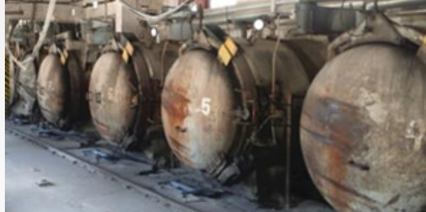
Figure 2: Autoclaves in Ludynia H+H Silicaty, (near Kielce).
